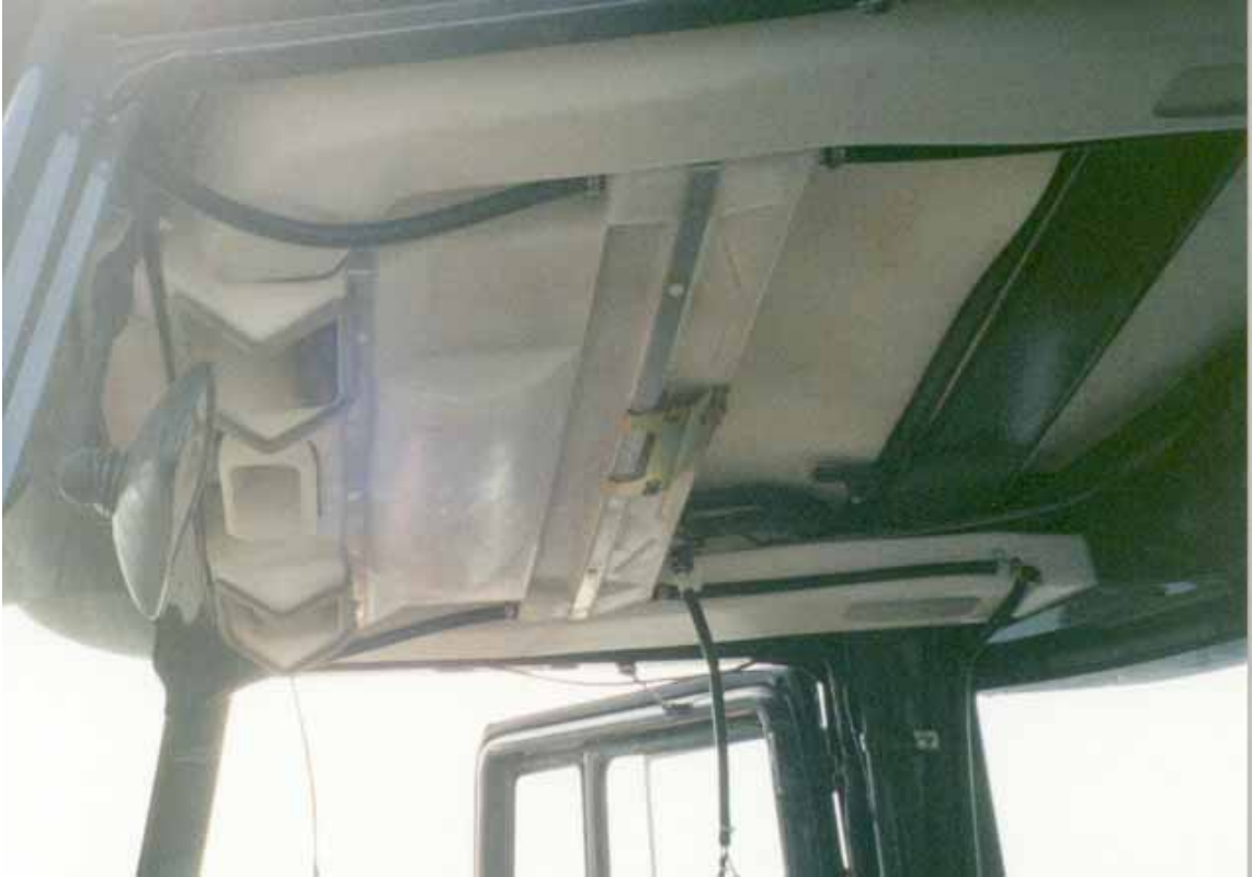
Drain lines (4) running front and back. Down corner posts at front and down side columns at rear.
