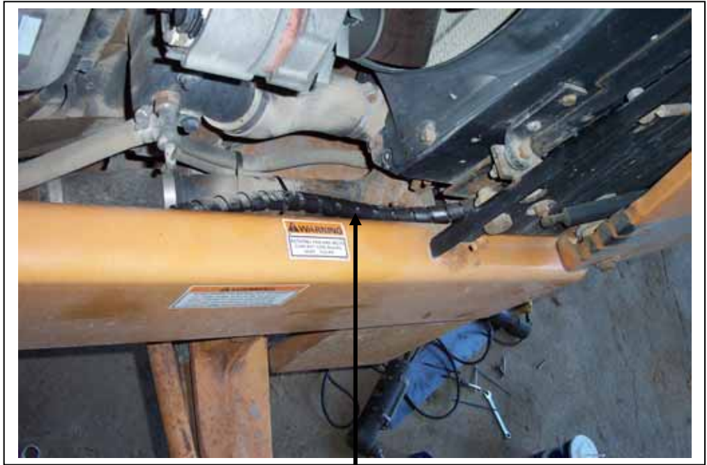
5/16" line from condenser to drier
