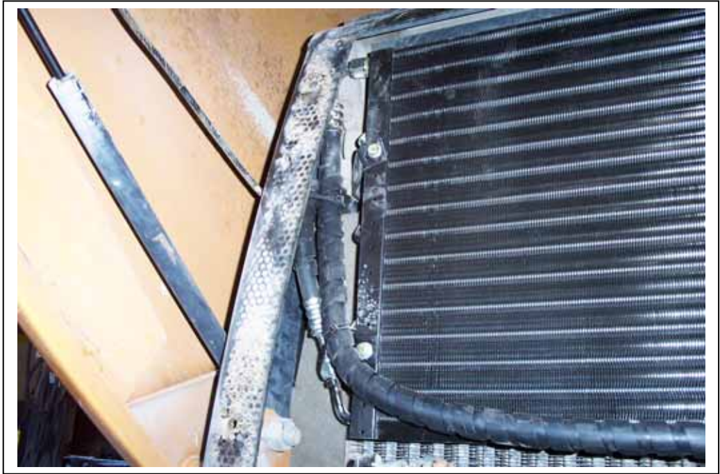
Hose runs at the condenser
